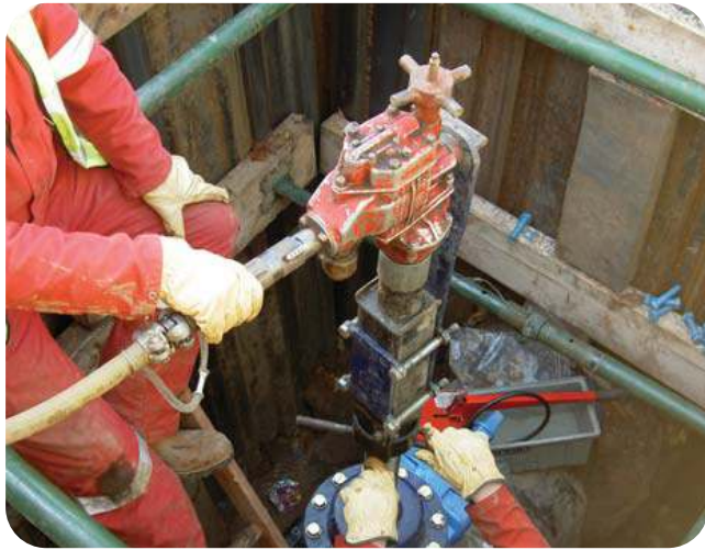
All installations are carried out by fully trained City and Guilds operatives
