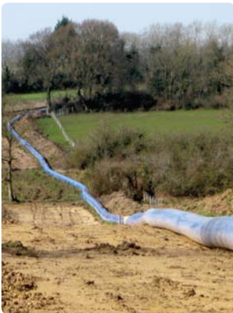
One of Radius Systems' factories in Northern Ireland will be supplying pipes for this prestigious project
