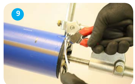
9 To prevent the swarf contaminating the pipe, cut using the round nose snips at regular intervals
