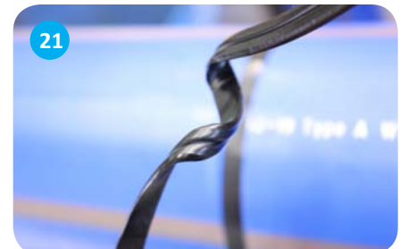
21 Assess the joint by checking the bead quality and carrying out a bend back test. If the bead is defective, cut-out and remake the joint
