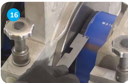
16 Check the min and max exposed core pipe distance tolerance after trimming. Ensure no contaminants come into contact with the prepared pipe ends
