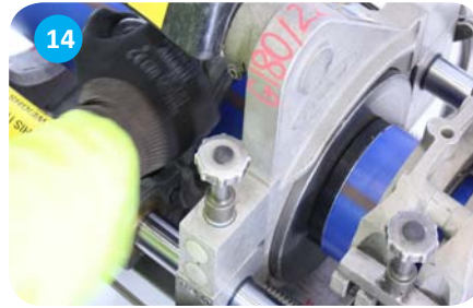
14 Follow water industry standard butt-fusion procedure. Program the butt-fusion unit with the correct Puriton pipe parameters: diameter, water PE100 pipe, SDR17
