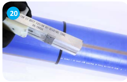
20 Allow the joint to cool in the butt-fusion unit. Once cooled remove the bead using a de-beading tool
